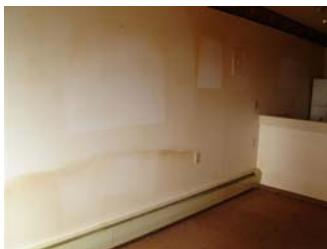
Residue on Walls
