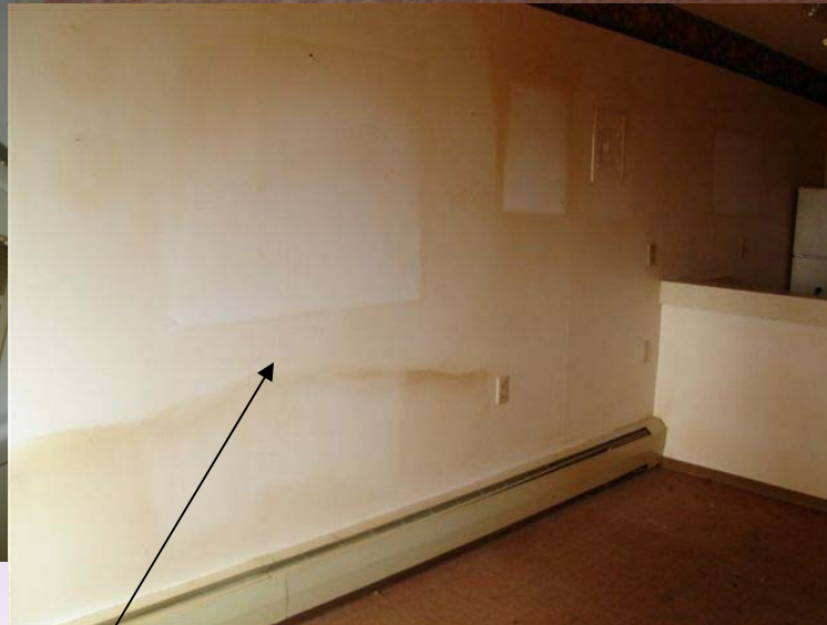
Residue on Walls
