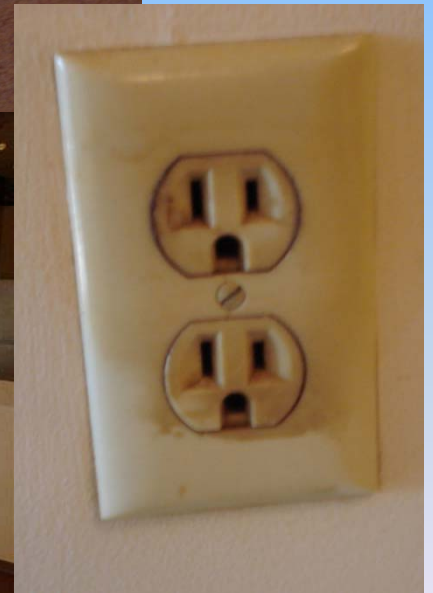
Residue on Electrical Outlet
