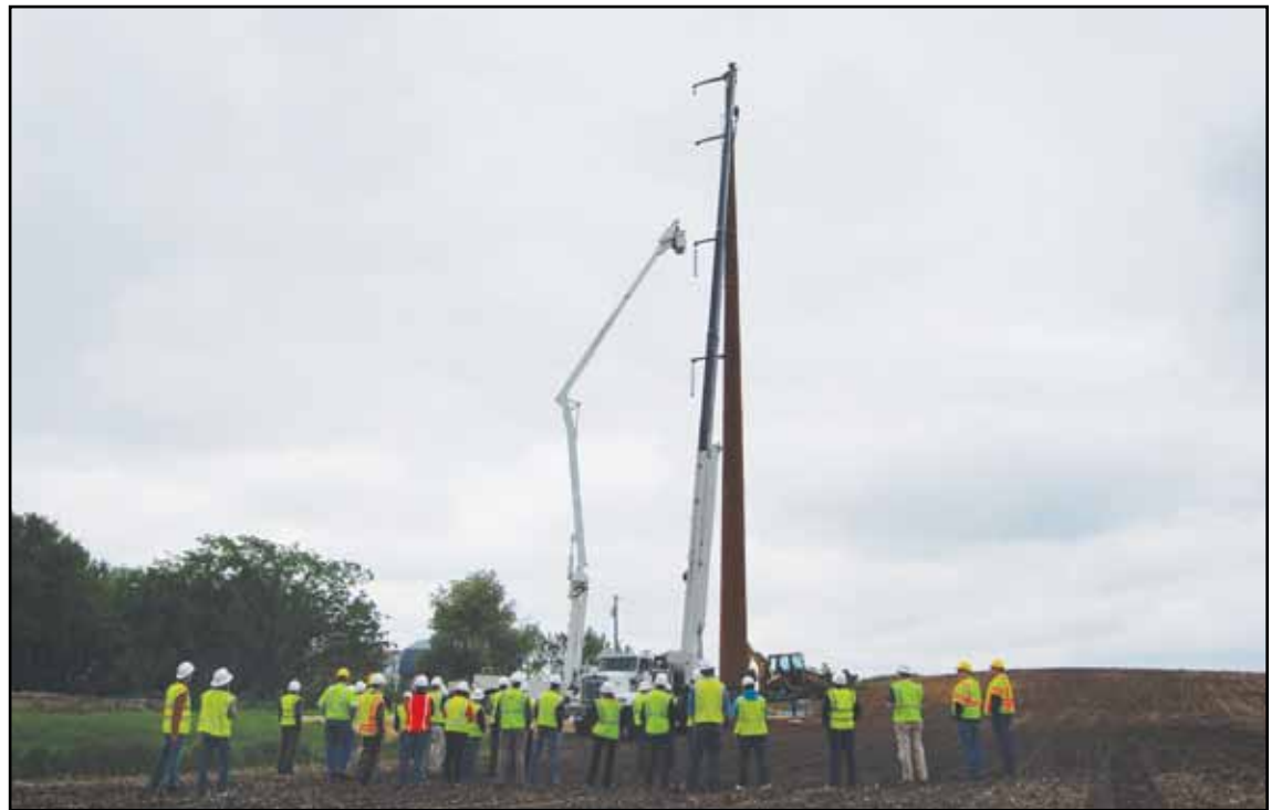
Construction of electric transmission lines has been a fairly common sight throughout Minnesota the past couple years. This was the scene June 7 north of Rochester, as a pole in a 161-kV line that will eventually connect to the Rochester Public Utilities system was set in place.
